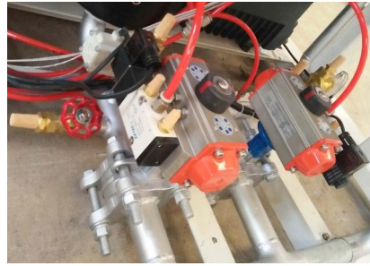
Vacuum Control System
